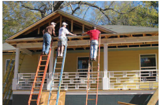
Fannie Mae employees participate in a home build project with Habitat for Humanity.
